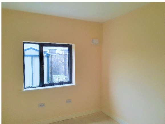
Wall-mounted humidity sensitive air inlets were used in the living rooms and bedrooms.
