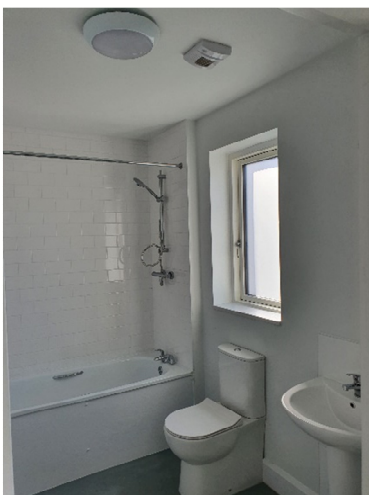
Demand controlled exhaust units were used in the bathrooms, Kitchen and Utility rooms. They provide the right amount of exhaust ventilation and are connected to the V4A fan
