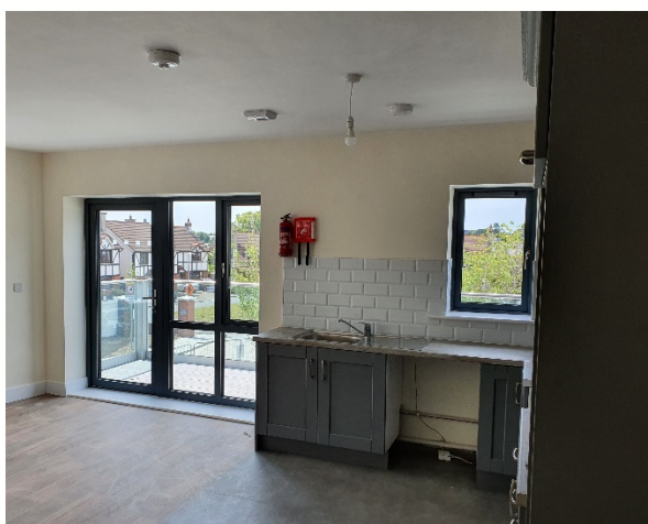
Demand controlled exhaust units were used in the bathrooms, Kitchen and Utility rooms. They provide the right amount of exhaust ventilation and are connected to the V4A fan
