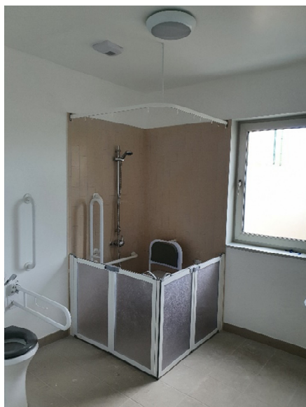
Demand controlled exhaust units were used in the bathrooms, Kitchen and Utility rooms. They provide the right amount of exhaust ventilation and are connected to the V4A fan
