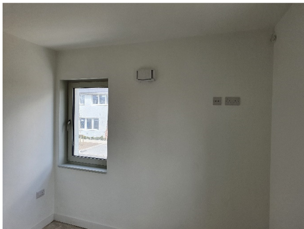
Wall-mounted humidity sensitive air inlets were used in the living rooms and bedrooms.
